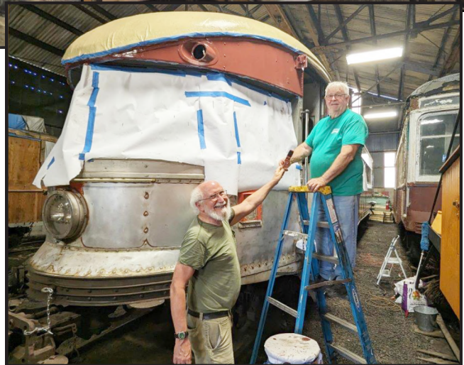
Top left: Volunteer Fred Walter has worked on numerous projects in his 58 years of volunteering at RTM. Here, he is repairing the DC welder on work car 64.
