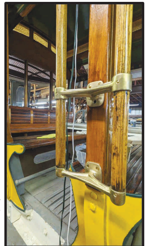
Right: 1875's newly sanded and varnished grab bars after being reinstalled. The brass hardware has also been polished.
